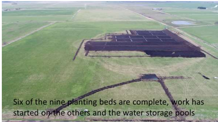
13 Aerial shot of planting beds, partly finished, partly still in construction (Photo: Henry Stanier)
